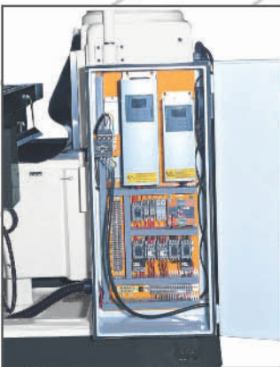
Electric box with inverters
